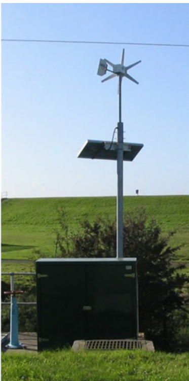
A low energy remote power site where a grid connection would otherwise cost thousands of pounds
